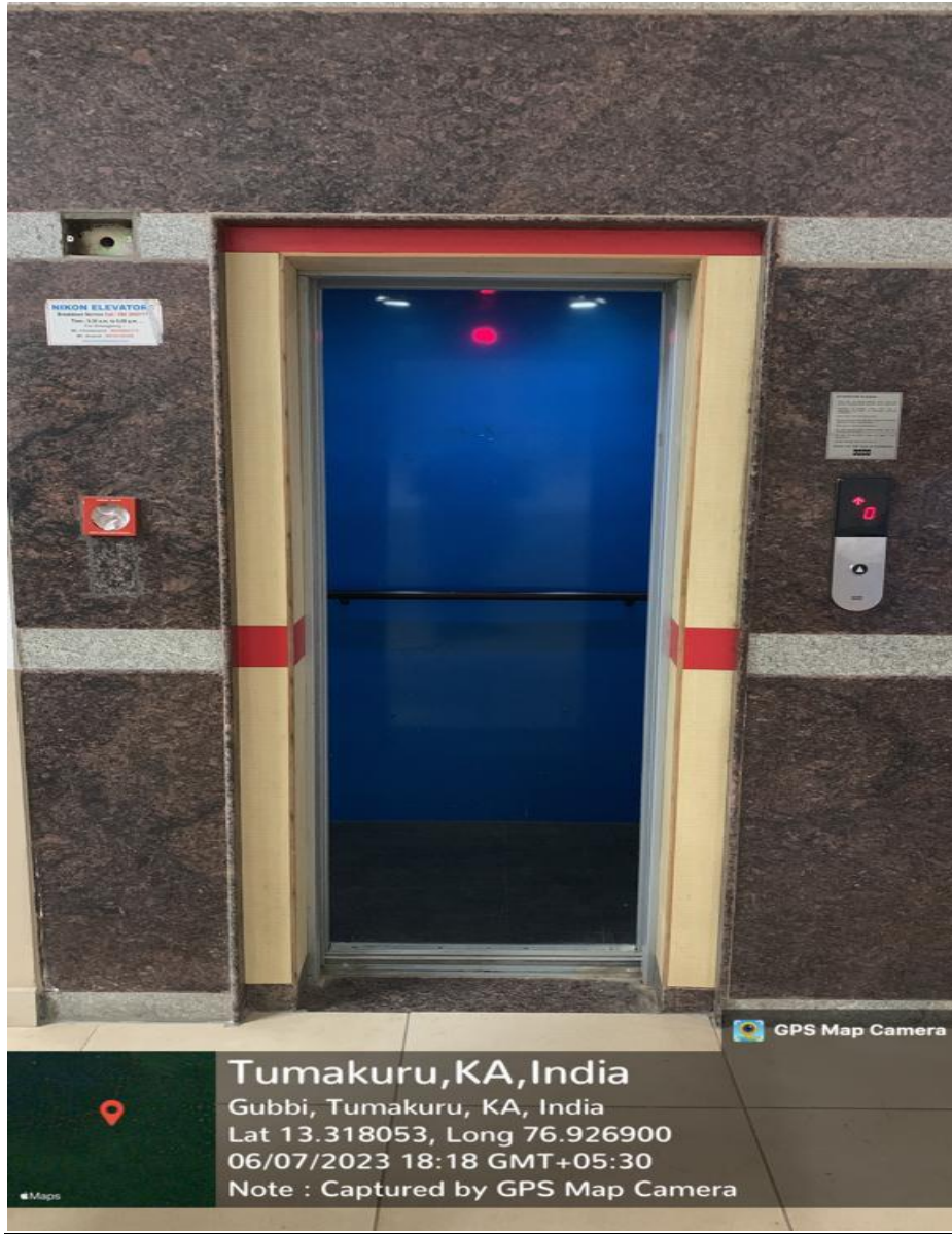
Lift in Admin Block
